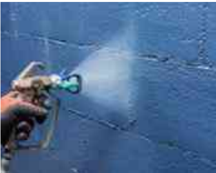
... unplastered walls, and
